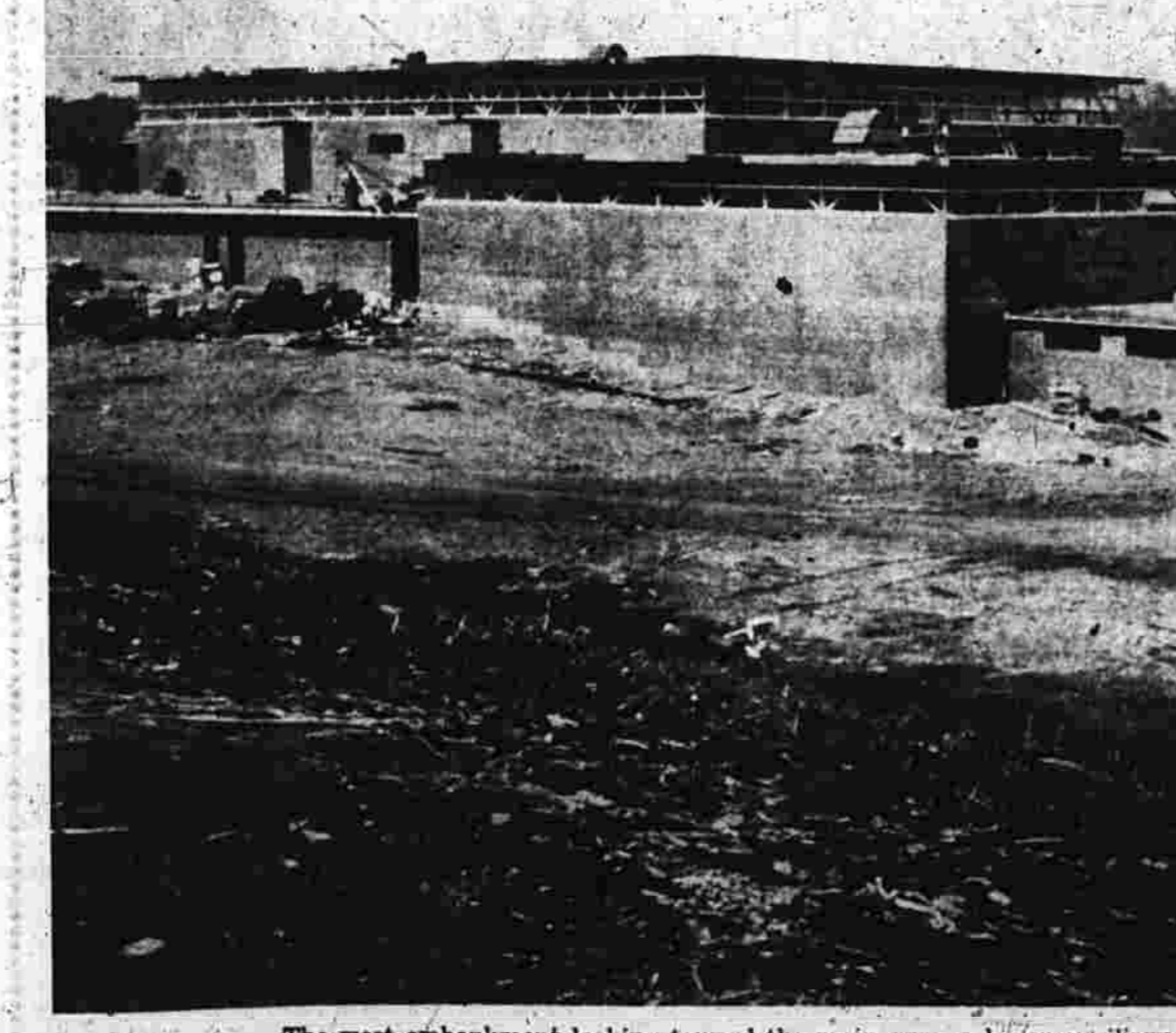
The west embankment looking toward the main gym, a lower auxiliary gym and the swimming pool.
