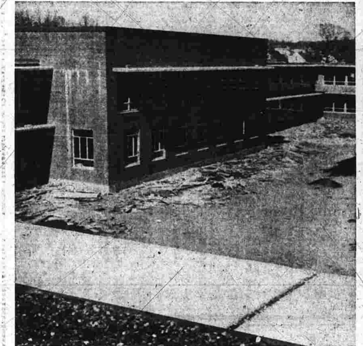
The roof over the shops looking at the quadrangle side of the administrative wing.
